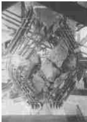
Figure 2-20 Shear failure of La Cienega-Venice Undercrossing Collector Distributor 36 possibly caused by axial tension (Papazoglou and Elnashai 1996).
