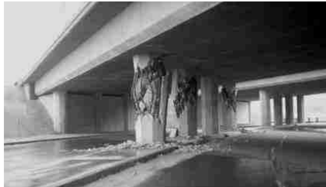
Figure 2-18 Column failure of Foothill Boulevard Undercrossing caused by effects of skewed superstructure (Earthquake Engineering Research Center, University of California-Berkeley).
