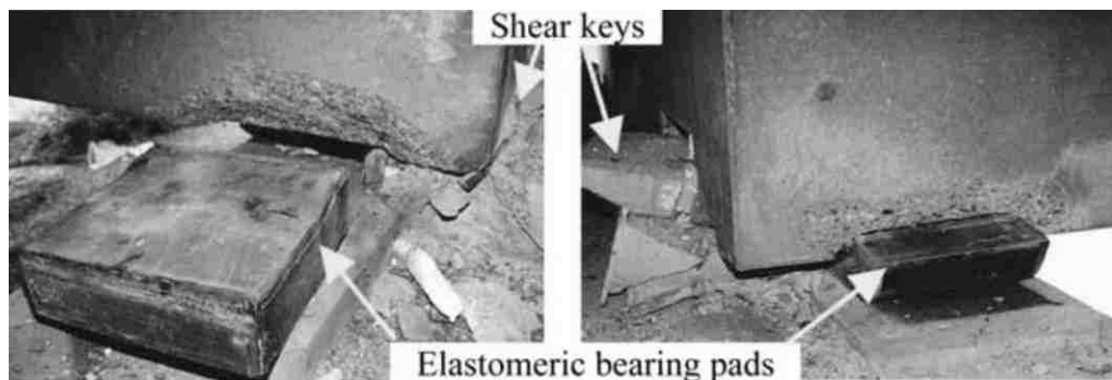
Figure 2-5 Sliding failure of bearing pads (Pamuk et al. 2005).
