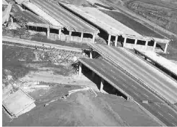
Figure 2-4 Superstructure failure due to unseating (Andrawes and DesRoche 2005).
